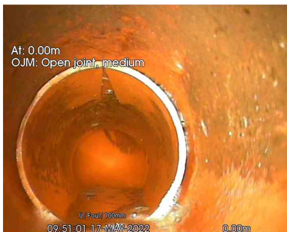
SVP_0-00m_095101.jpg, 00:00:16, 0.00 m Open joint, medium
