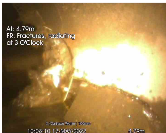
GY1_4-79m_100810.jpg, 00:01:21, 4.79 m Fractures, radiating at 3 o'clock
