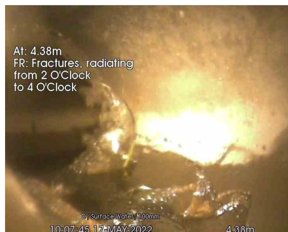
GY1_4-38m_100745.jpg, 00:01:04, 4.38 m Fractures, radiating from 2 o'clock to 4 o'clock
