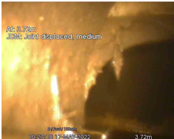
GY3_3-72m_102718.jpg, 00:00:55, 3.72 m Joint displaced, medium
