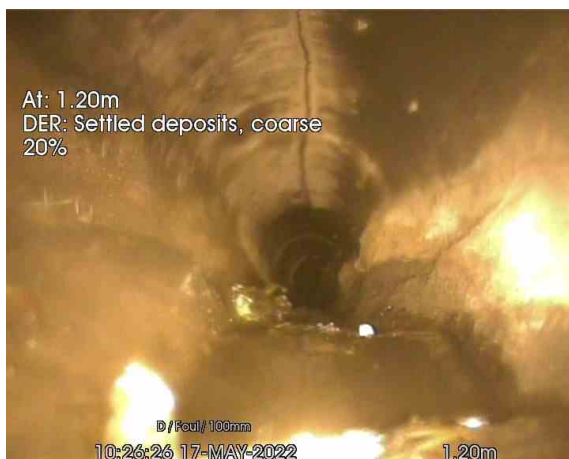
GY3_1-20m_102626.jpg, 00:00:16, 1.20 m Settled deposits, coarse, 20% cross-sectional area loss
